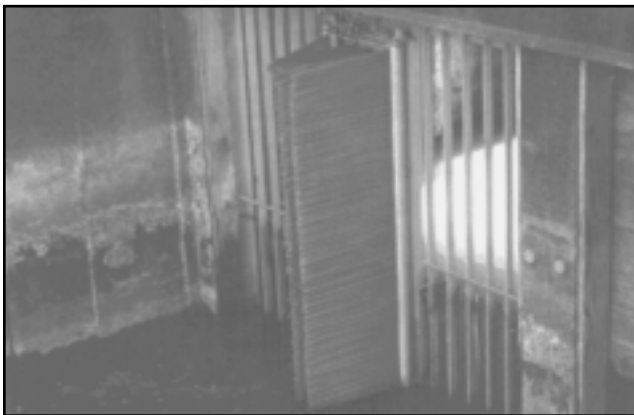
This structure can be opened to allow native fish into the floodplains, then closed to exclude carp later on.
