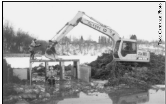
The water and fish control structure is installed in the Sunfish Pond Christmas tree enclosure.
